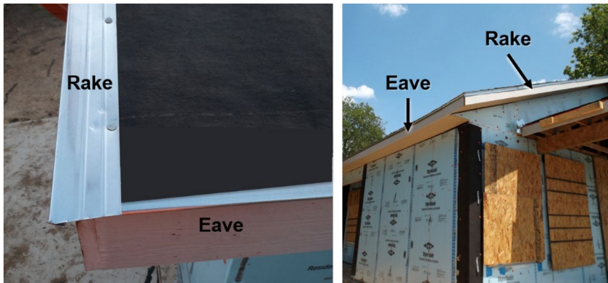
Figure 8-3. Felt Paper Goes Over the Drip Eave Along Eaves and Under Along Rakes
