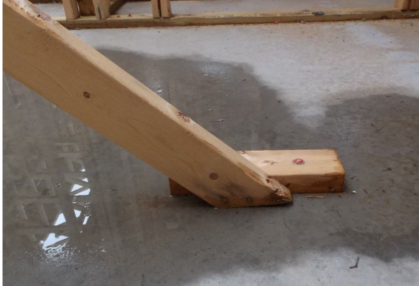
Figure 4-11. Do Not Use Blocks to Anchor Wall Bracing
