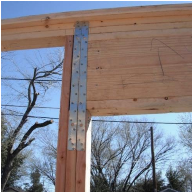
Figure 4-19. Hurricane Strapping on Garage Door Wall
