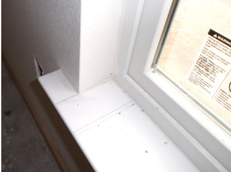
Figure 12-19. Notched Window Sill
