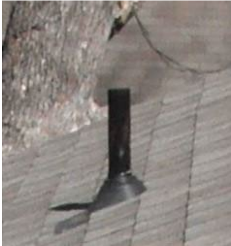
Figure 8-34. Paint Vent Pipes
