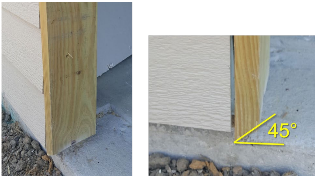
Figure 9-34. Bottom of Ripped 2x8 Around Garage Door Opening
